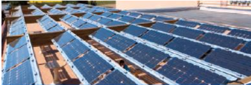
SOLAR PERGOLA AT THE LACQ SITE.
