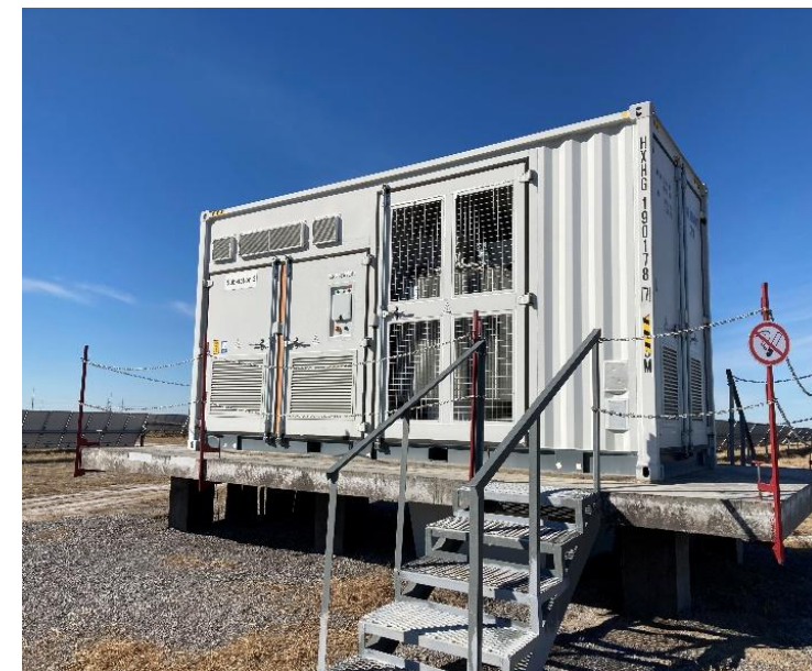
One substation Sungrow inverter
