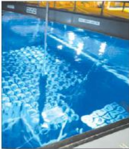
Typical spent nuclear fuel storage pool.
